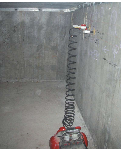
Figure 4. Equipment used to pressurize tendons and find the source of water.
