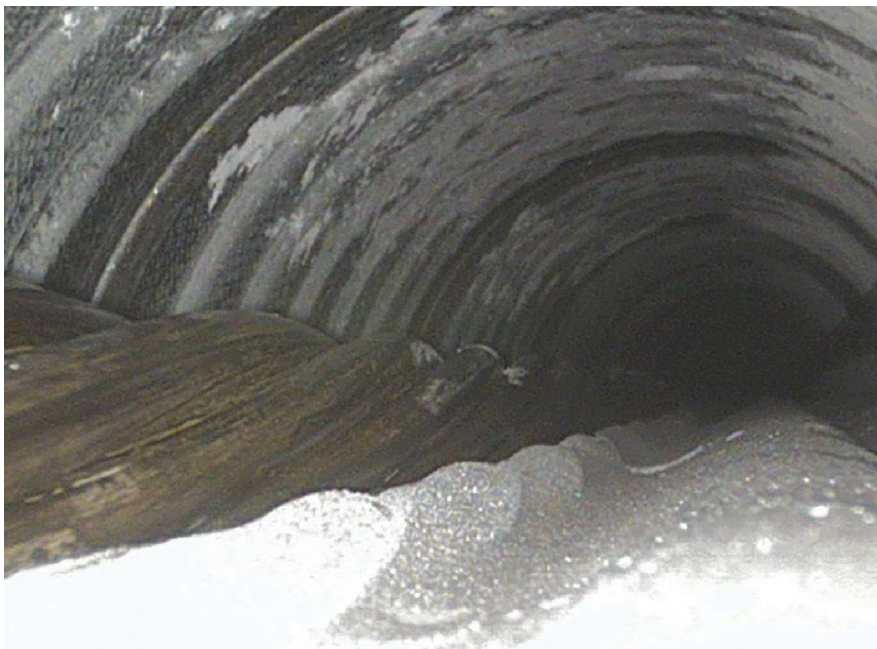
Figure 1. Bare strand in a tendon at a grout void. All Figures: Bruce Osborn.
