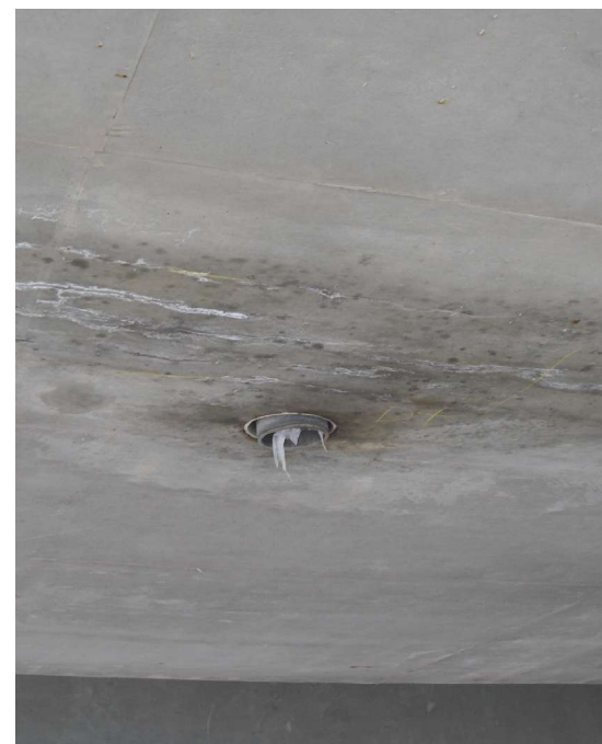
Figure 5. Signs of tendon corrosion near a bridge drainage system.
