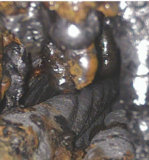
Figure 2. Bare strand with clear signs of corrosion in a tendon with a grout void.
