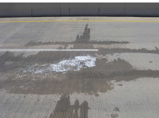
Figure 3. Operation to find cracks in the bridge that were leading to moisture in post-tensioned tendons.
