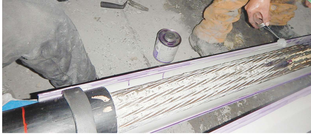
Installation of a split-duct system for permanent repair of external tendons for the Y Interchange project in San Antonio, Tex.
