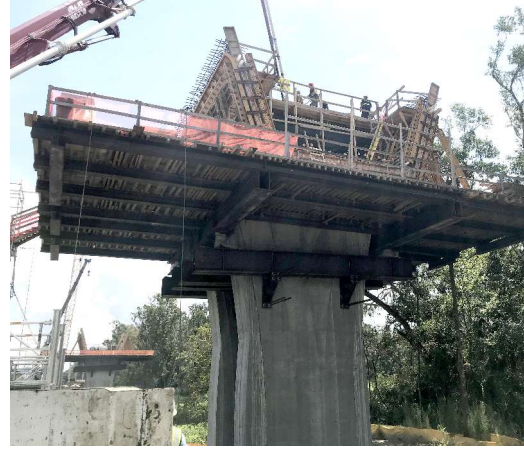
For the Wekiva Parkway pier table, three-dimensional component models were used to facilitate reinforcement placement. Photo: FINLEY Engineering Group.
