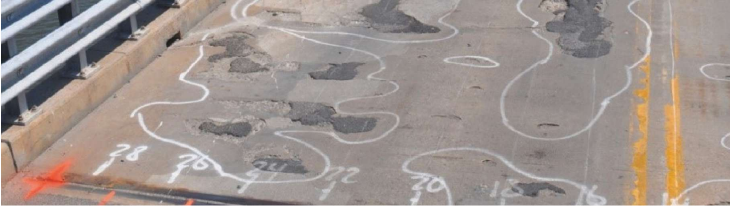
Example of a concrete bridge deck in poor condition. Photo: Dr. Thomas Schumacher.
