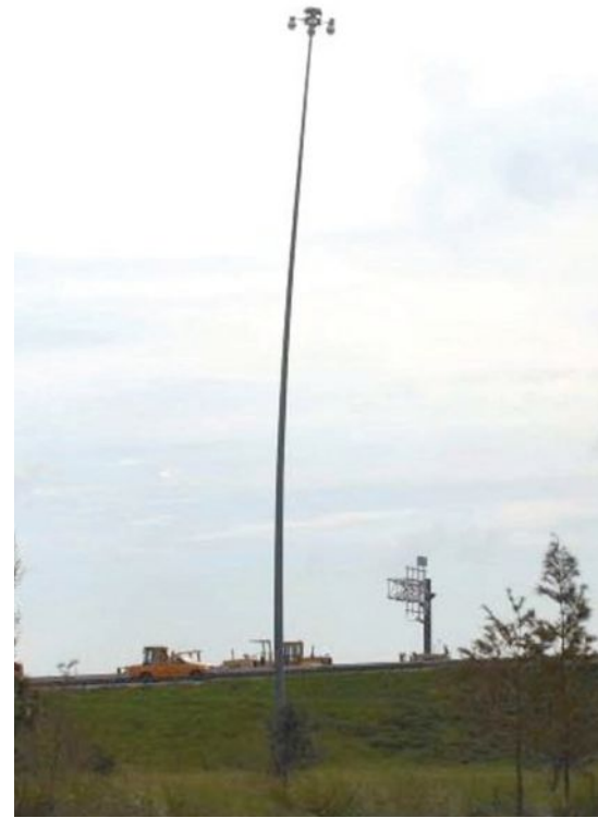
Figure 1. Florida Department of Transportation photo showing high-mast illumination pole during a high wind. All Photos adapted from Reference 2.
