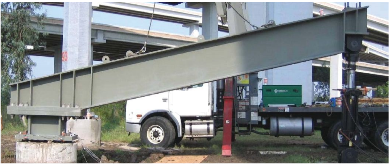
Figure 3. Setup for field testing the deep anchors in the ASR-damaged drilled-shaft foundation of a high-mast illumination pole.
