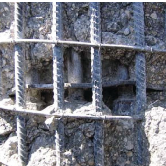
Figure 4. No corrosion of the reinforcement was evident in the drilled shafts having significant cracks likely caused by ASR.
