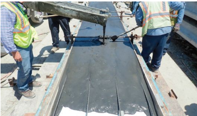
Figure 4. Construction of 60-ft-long voided box beam using an ultra-high-performance concrete mixture developed using the approach outlined in the draft guidelines for production included in the Phase I report of the PCI-funded study. Photo: Wiss, Janney, Elstner Associates Inc.
