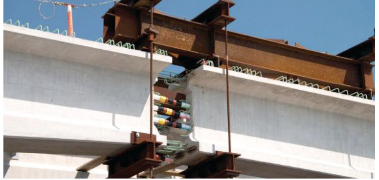
A close-up view of the strongback supporting the end segments on the pier segments before the closure pour. Spliced post-tensioning ducts are visible in the 24-in.-wide joint. Stirrups and other closure pour reinforcement had not yet been installed. Photo: R.E. Pierson Construction Company.
