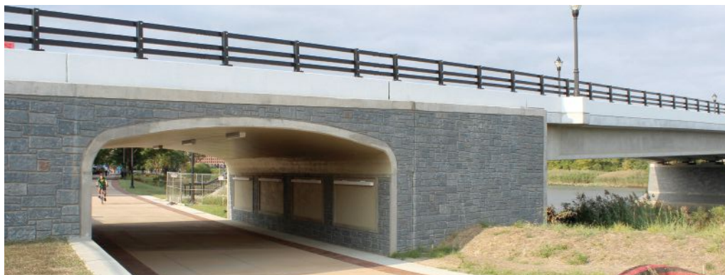
View of the completed underpass for the shared-use path. Panels for future displays of artwork are visible on the walls of the underpass. Photo: Robert J. Healy.
