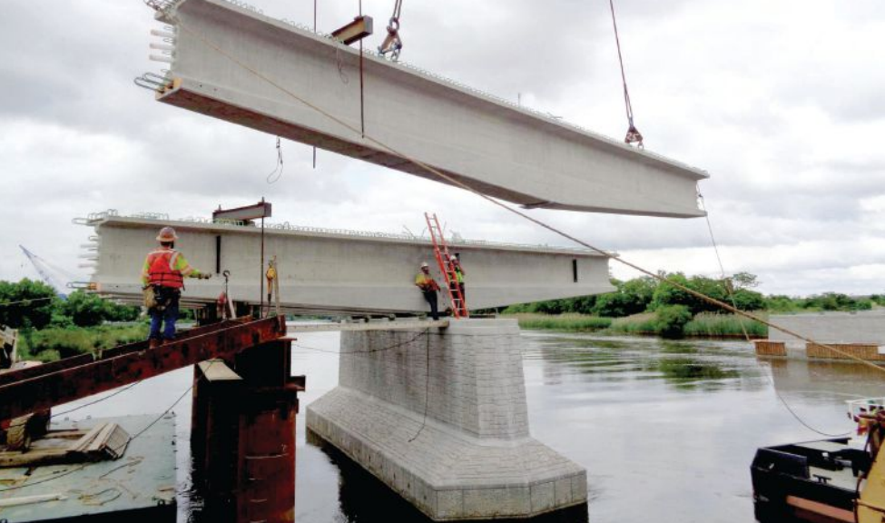
Erection of a haunched pier segment at pier 1. Note the temporary bent in the river being used to temporarily support pier segments. Photo: R.E. Pierson Construction Company.
