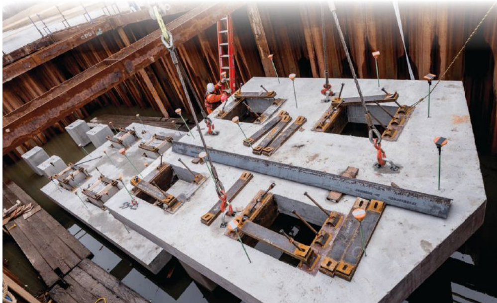
Cofferdam at bridge pier 2 showing 30-in.-square concrete piles and one of the precast concrete bottom soffit form slab segments being placed. Photo: R.E. Pierson Construction Company.
