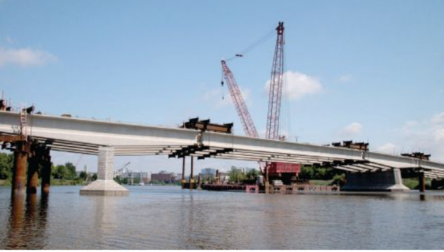
With all concrete girder segments erected, strongbacks temporarily support girder segments until closure pours and post-tensioning are completed. Photo: R.E. Pierson Construction Company.
