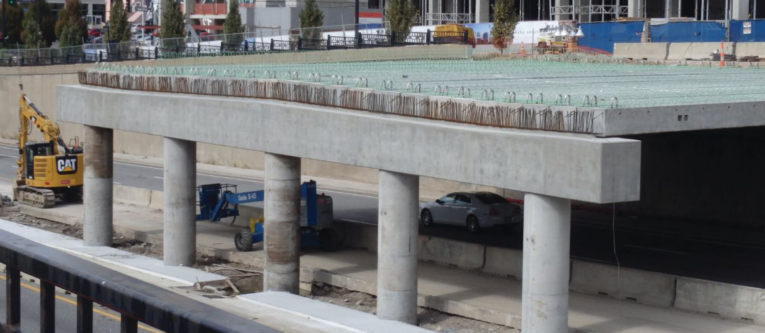
Erection of one span of prestressed concrete box beams for the Grand Boulevard Bridge. The reverse crown in the cross section and pier cap is visible.
