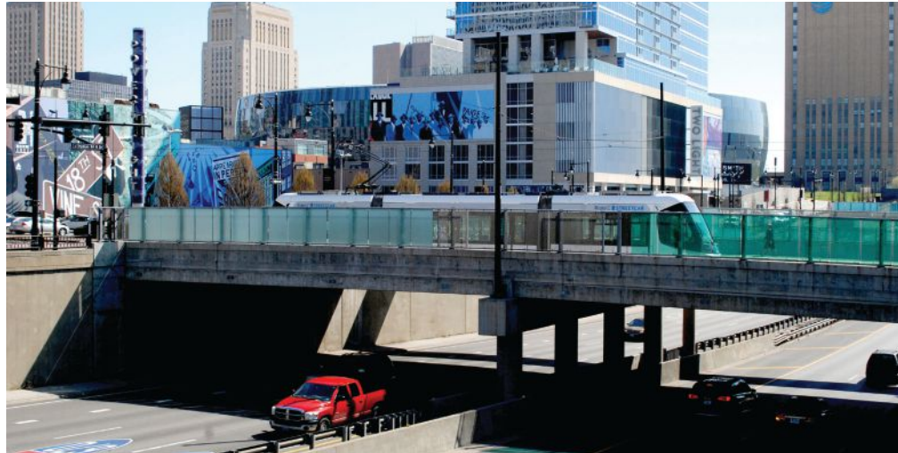
Elevation view of the Main Street Bridge. Note that a streetcar is crossing the bridge. All Photos and Figures: HDR.
