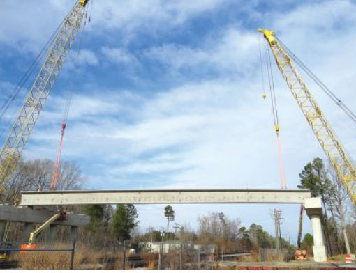
Dual crane setting operation for the 85-in.-deep, 156-ft 2-in.-long prestressed lightweight concrete bulb-tee beams spanning over the CSX Transportation railroad. Clips on the beam web were for crossframes and utility hangers for conduits.. Photo: Whitman, Requardt & Associates.
