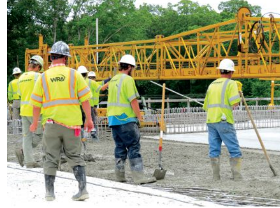
Lightweight concrete being placed in the deck. VDOT Class III (stainless steel) reinforcement was used in the concrete deck and barriers. Photo: Whitman, Requardt & Associates.
