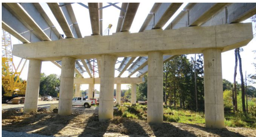
View of a typical pier near the middle of the bridge showing prestressed concrete beams before deck placement. The 12-span structure has 11 five-column concrete piers that reach up to 40 ft tall. The piers are supported by 520 plumb 16-in.-square prestressed concrete piles totaling over 27,000 linear feet. Photo: Whitman, Requardt & Associates.
