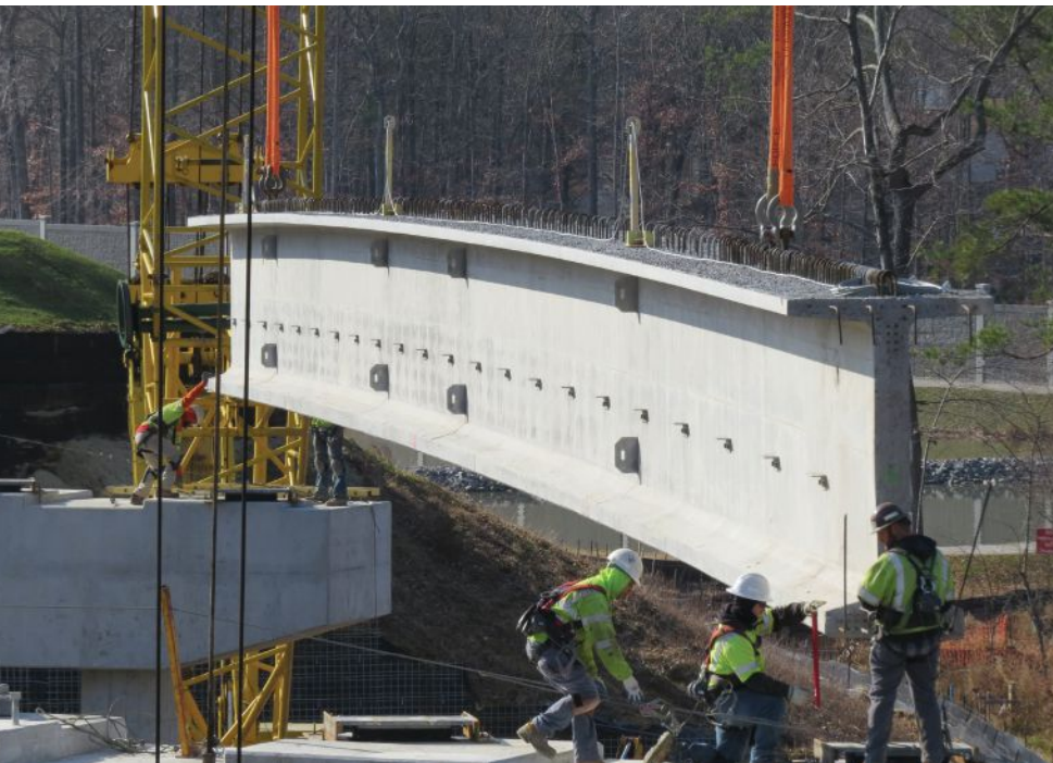
View of 155-ft-long, 85-in.-deep prestressed concrete bulb-tee beams during the setting operation. Beam camber was a major concern due to the long times between beam production and erection. This concern was mitigated using time-dependent methods to recalculate the predicted camber and adjust the substructure seat elevations. As a result of the contractor and fabricator working directly with the design engineer, the camber predictions were a good estimate of the actual field-measured camber. Photo: Whitman, Requardt & Associates.
