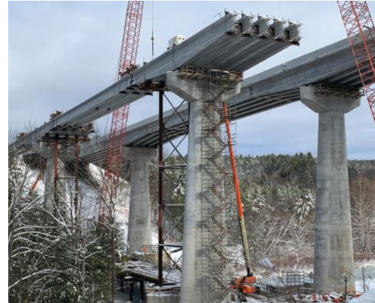
Construction of the southbound bridge superstructure with the completed northbound bridge in the background.
