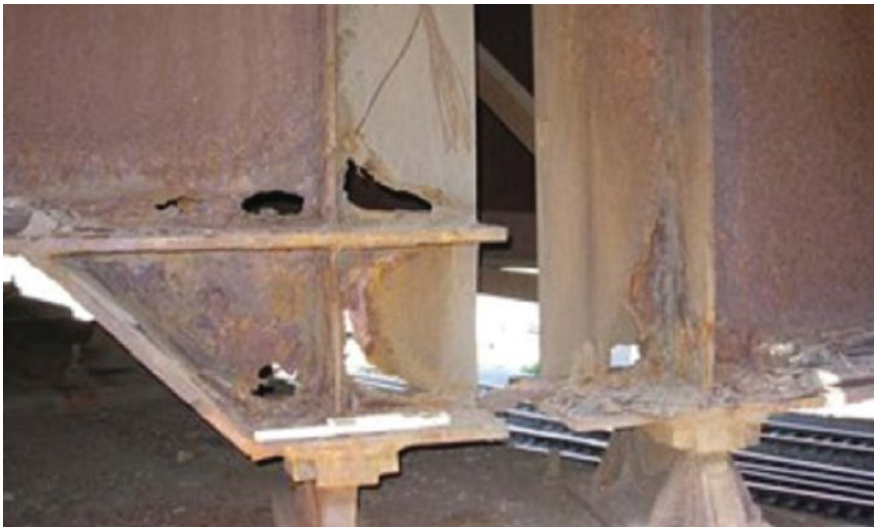
Figure 1. Leakage from failed or deteriorated bridge deck expansion joints can cause deterioration of beam ends, bearings, and substructure elements. All Photos and Figures: Federal Highway Administration.
