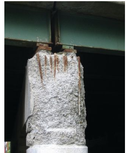
Figure 2. Chemical-laden surface runoff can accelerate substructure deterioration beneath an expansion joint.
