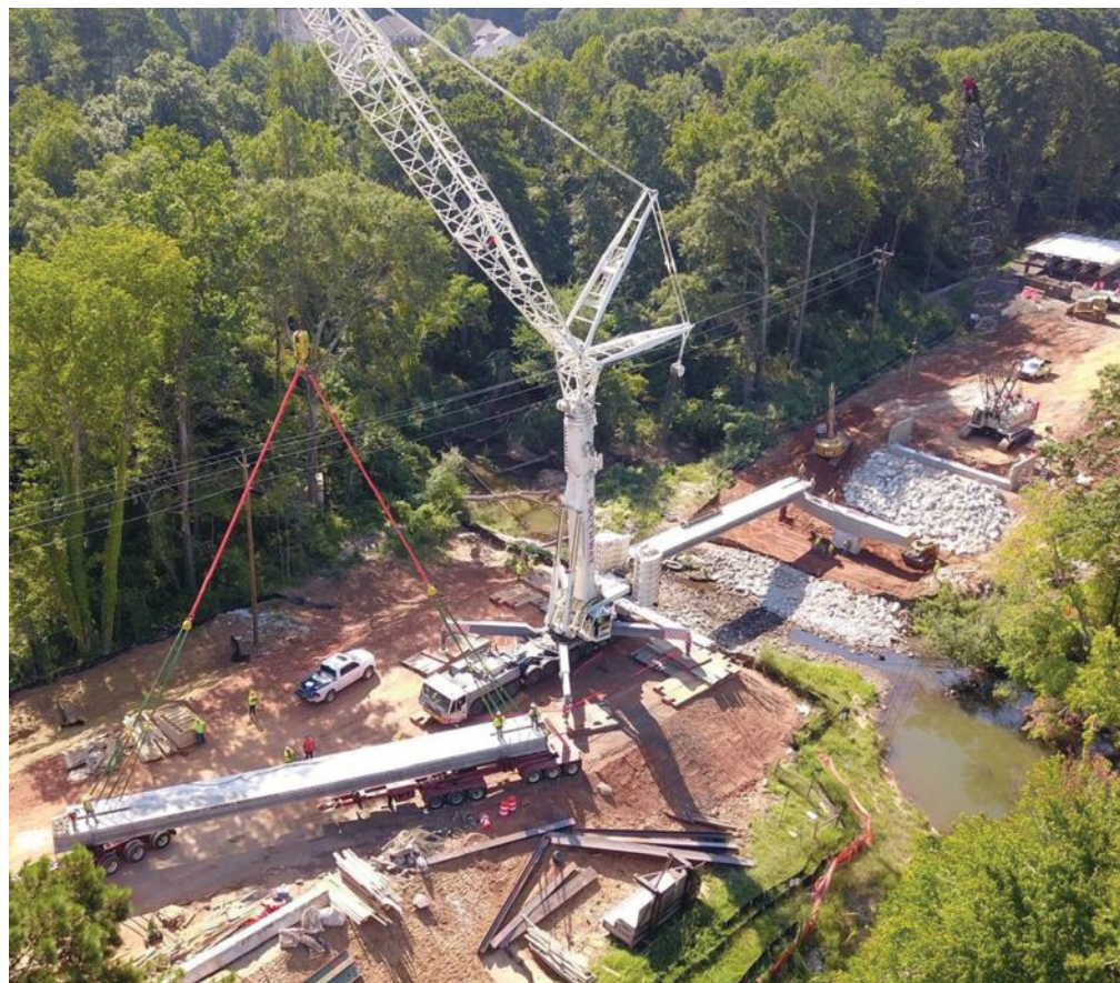
An 800-ton crane placing a 93-ft-long decked beam unit for the main span. Photo: C.W. Matthews Contracting Co. Inc.
