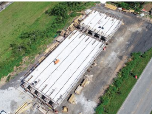
Aerial view of the on-site staging area showing completed decked beam units for spans 2 and 3. Photo: C.W. Matthews Contracting Co. Inc.
