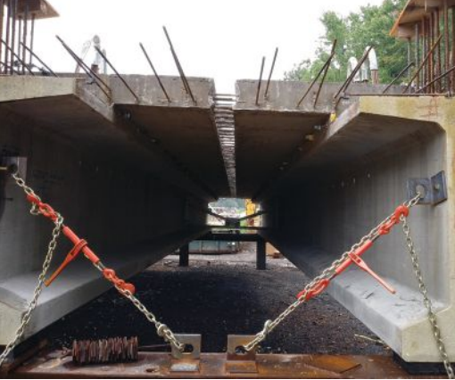
Completed decked beam units in the staging area. The bracing can be seen in the background. Photo: CHA Consulting.
