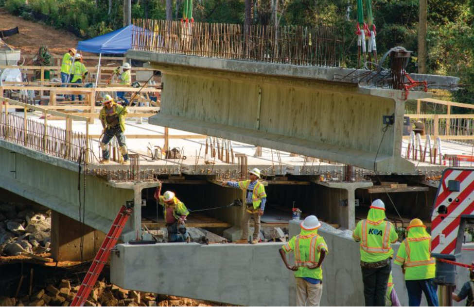
Decked beam unit being erected into final location at end span. Photo: CHA Consulting.
