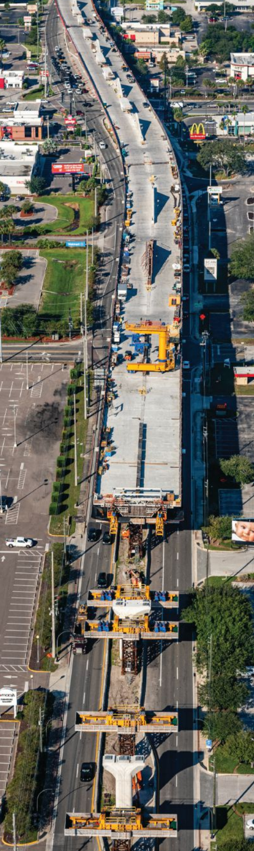
Photograph showing stages of construction of finback structure of the Selmon West Extension. Temporary shoring towers to allow erection of the next section of the bridge using the progressive span-by-span method are shown in the foreground. Several spans with their finbacks are visible in the background. Photo: Tampa Hillsborough Expressway Authority.
