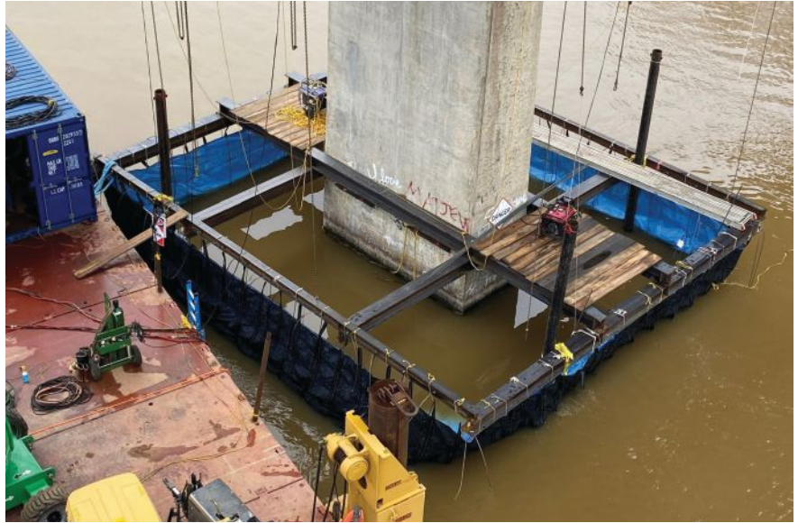
The North Carolina Department of Transportation approved the fabric concrete forming system using multiple layers of reinforced proprietary geotextile fabric developed by TrapBag Barrier Systems for the repair of a footing for the Lake Tillery Bridge rehabilitation project. All Photos: PCL Construction.
