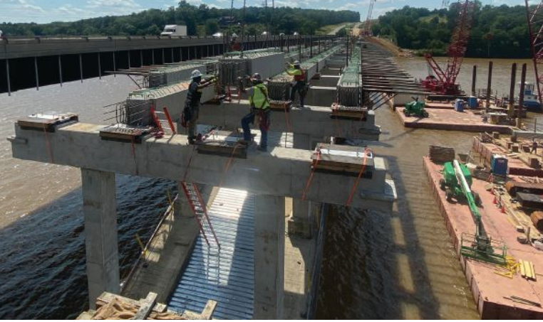
New precast concrete box beams are erected in span F. Note the continuity reinforcement detail at the beam end, the common bearing under the continuity diaphragm, and the epoxy-coated reinforcement that will be cast into the composite deck.
