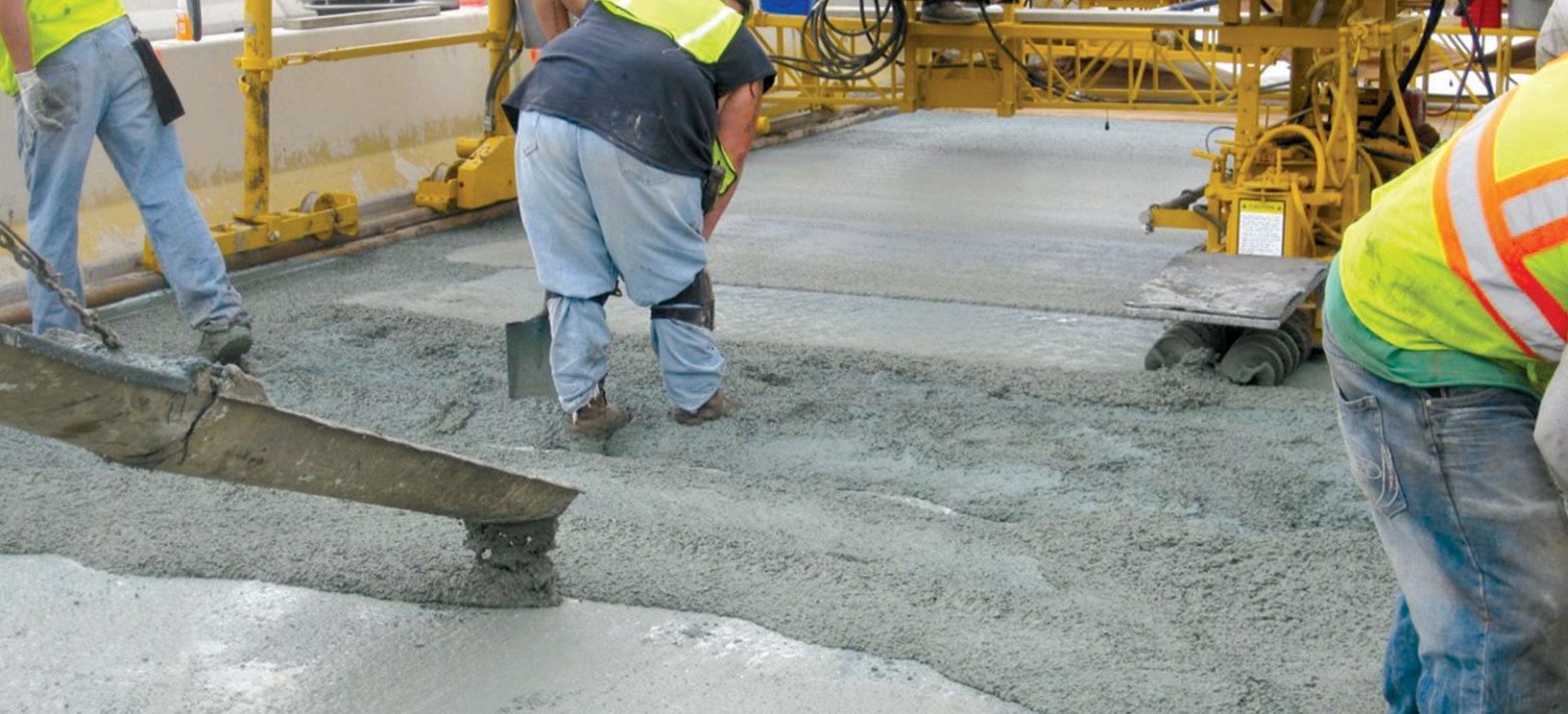
A crew places a latex-modified concrete overlay with good flow and consistency. All Photos: Pat Martens, Bridge Preservation & Inspection Services.
