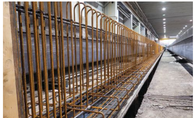
Following the installation of the stem welded wire reinforcement (WWR) in an inverted-tee section, the bottom-flange reinforcement is installed in the form of bent WWR mats.
