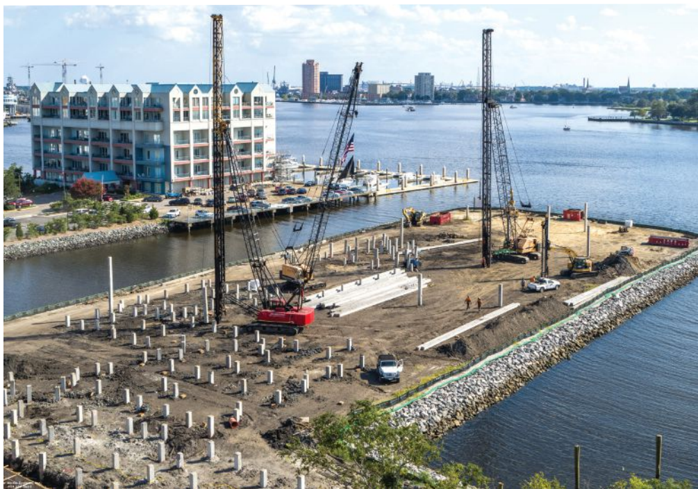
A typical on-land pile-driving operation allows piles to be stockpiled on site for easy access. Precast, prestressed concrete piles are displacement piles that create no spoil at the site. Photo: Concrete Technology Corp.
