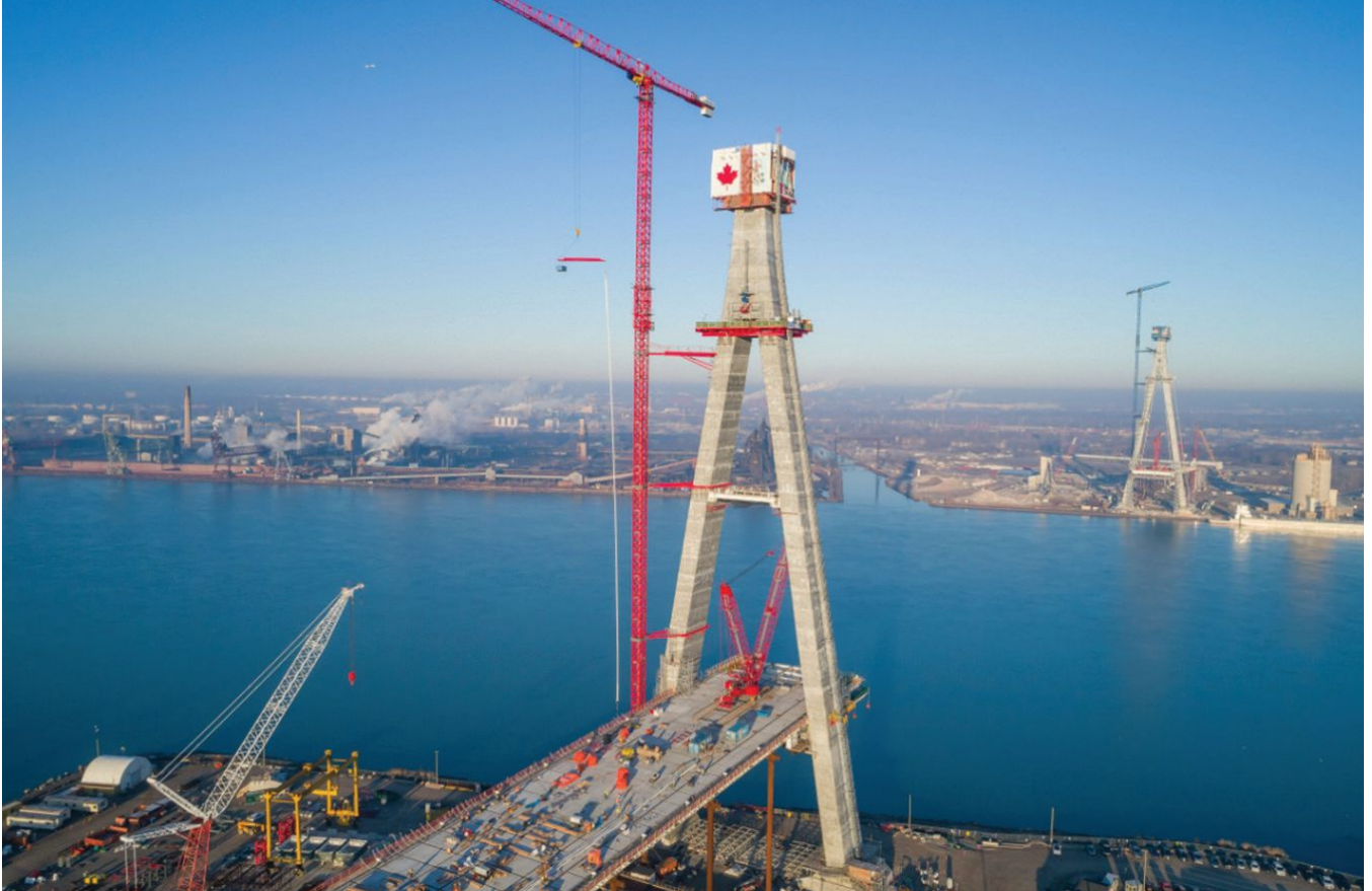
The two concrete towers, one in Windsor, Ontario, and the other in Detroit, Mich., for the Gordie Howe International Bridge are approximately 722 ft in height. Each tower is composed of two pylons, which give the structures the shape of an inverted “Y”. The top third of each tower houses the cable-stayed system that supports the bridge deck. Photo: Kelly McNutt Consultants.
