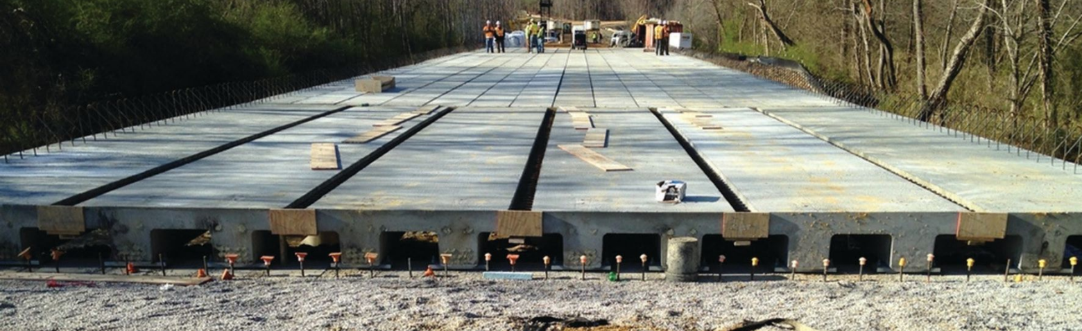
Secondary Route 770 Bridge over Hanging Rock Creek used modified Northeast Extreme Tee D beams (in foreground) in one end span; prestressed concrete cored slabs in the two center spans; and prestressed concrete solid slabs in the other end span. The structure is being monitored to evaluate the performance of the various types of beams and connection details.
