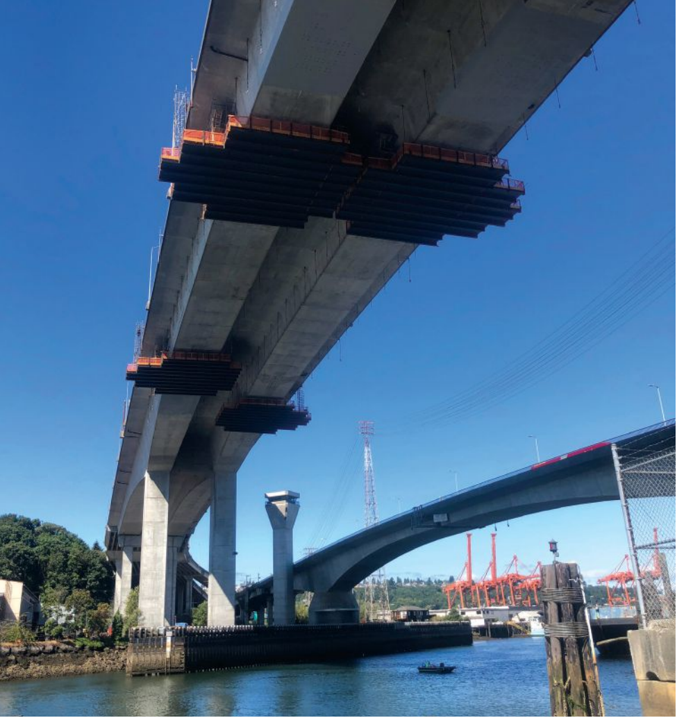
Kelly McNutt Consulting (KMC) worked with WSP on the emergency rehabilitation of the West Seattle Bridge in Seattle, Wash. KMC provided an independent construction estimate for the retrofit project. Photo: Kraemer North America.
