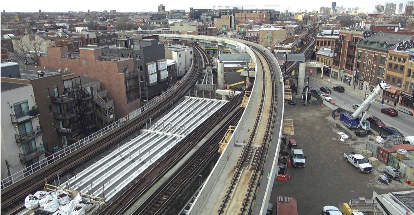
The north mainline construction for tracks 1 and 2 under the flyover structure. This view shows, from left, the temporary tracks; the precast, prestressed concrete beams that will carry tracks 1 and 2; tracks 3 and 4 on the existing structure; and the tracks on the flyover structure. Photo: Chicago Transit Authority.
