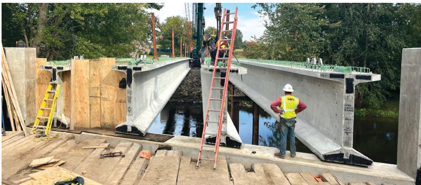
The 7-ft-deep prestressed concrete beams are among the largest in use in Michigan.
