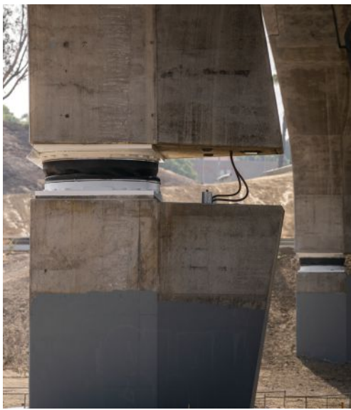
Because Isolation bearings are located within the vertical portion of the Y-bents, the team developed a new seismic isolation design methodology. Photo: HNTB, © Core-Visual.
