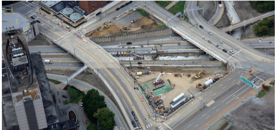
The site of the Interstate 579 Urban Open Space Cap project as construction begins, with the interstate highway running beneath. Photo: HDR Inc.
