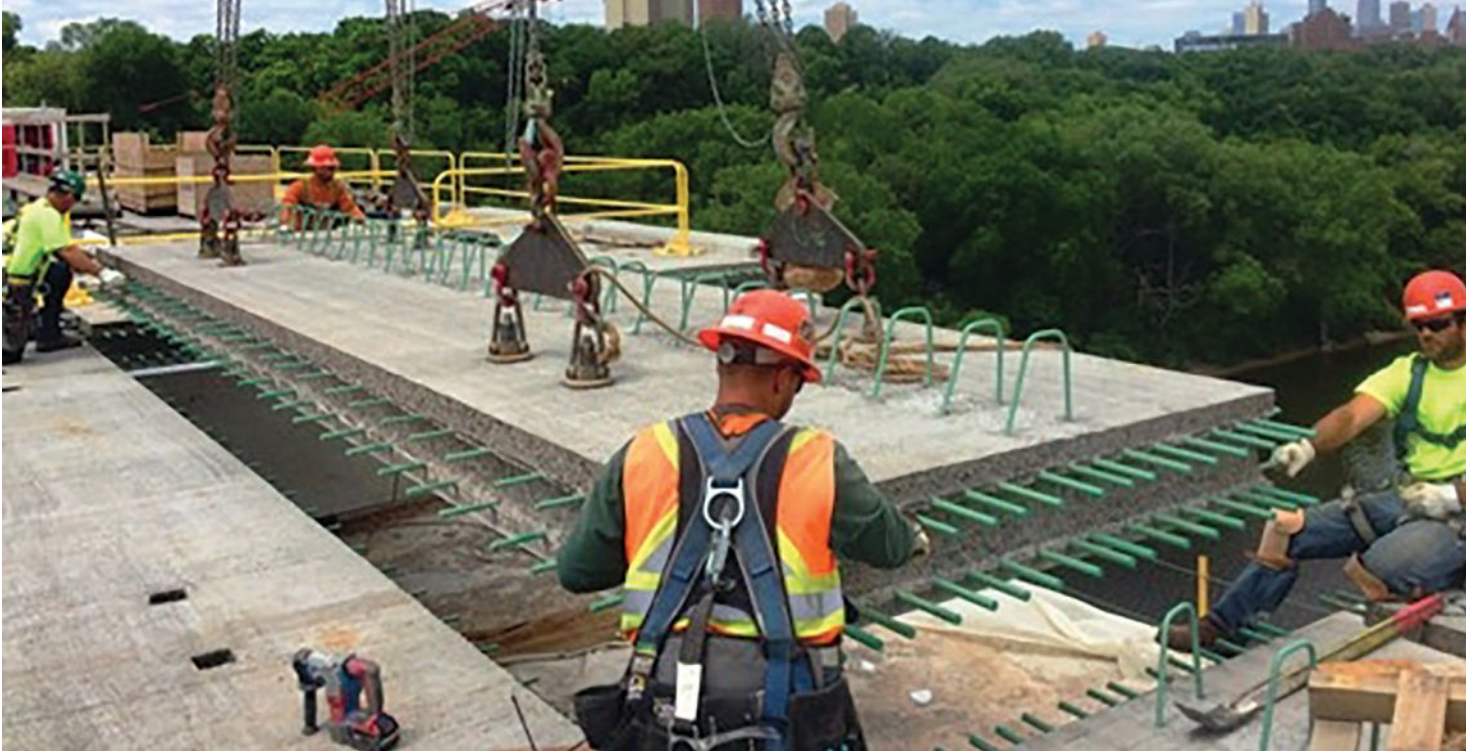
On the Franklin Avenue Bridge project in Minneapolis, Minn., Kraemer North America collaborated with others on the full removal and replacement of the superstructure beams and a complete replacement of the reinforced concrete bridge deck. Photo: HNTB.
