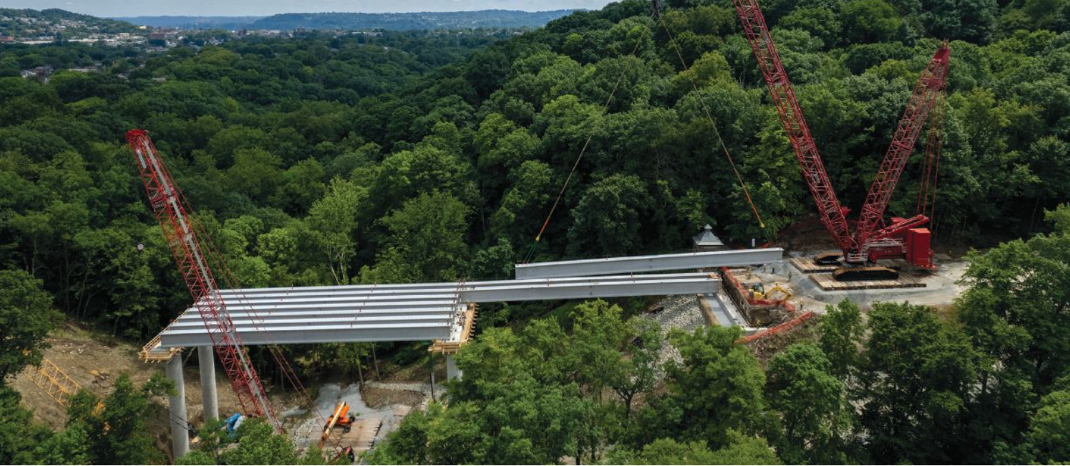
Cranes move the 200-kip, 154-ft-long prestressed concrete bulb-tee beams into position on the new Fern Hollow Bridge in late July 2022. Photo: Swank Construction Co.
