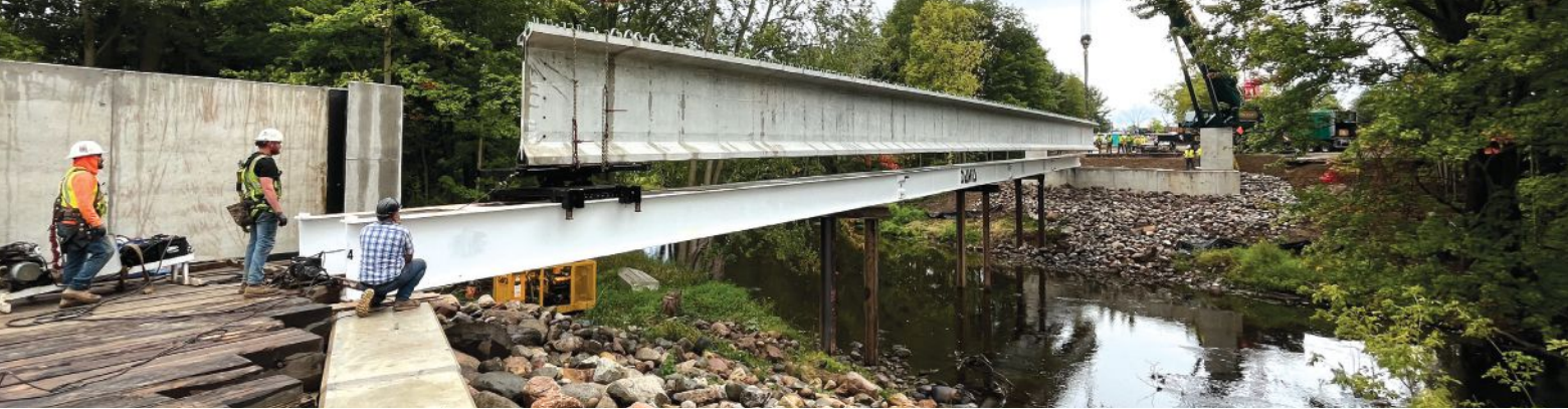
The first beam travels on the beam launcher. Once the beam is within reach of the crane on the opposite (east) side, both cranes set
