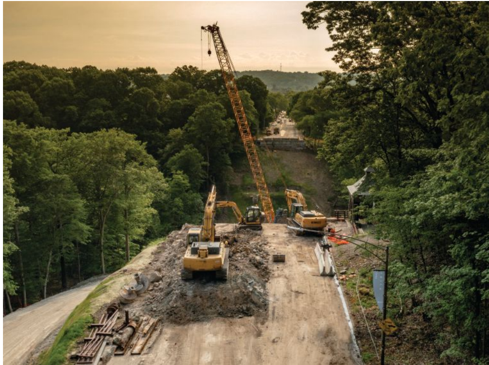
Site preparation work for the west approach to the new Fern Hollow Bridge in Pittsburgh, Pa., on the morning of June 1, 2022. Photo: HDR Inc.
