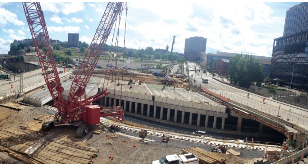
Some of the precast concrete adjacent box beams have been erected for three new bridge units between two existing bridges over Interstate 579. Photo: Pennsylvania Department of Transportation.
