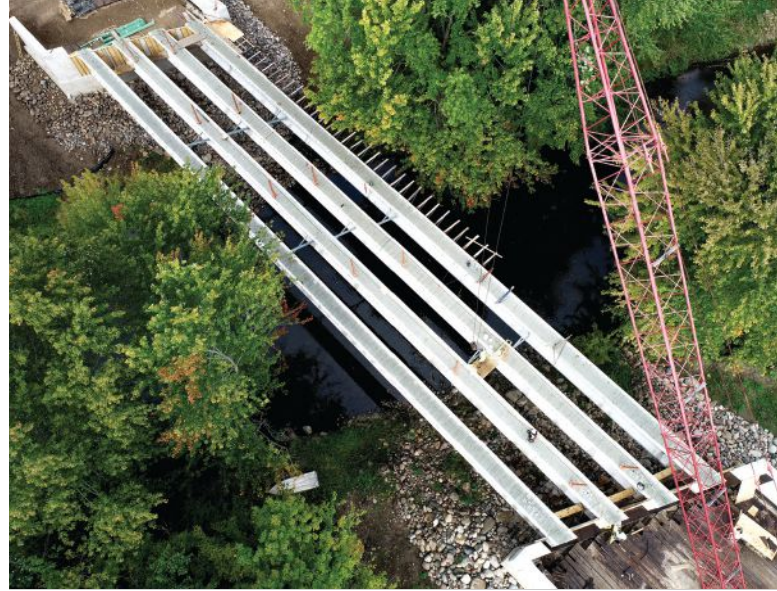
Aerial view of all four beams in place. The single-span solution eliminated six beams and a pier in the water.
