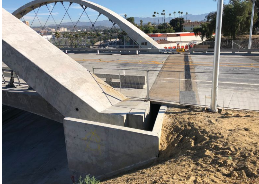
Steel plate expansion joints developed by the California Department of Transportation and modified for the viaduct are provided at each abutment, making the viaduct a 3058-ft-long continuous structure. The joints allow seismic movement of up to 30 in. in any direction. There is a sacrificial rubber seal at the back of each plate joint. Gaps to accommodate seismic movements can be seen between the arches and abutment. Photo: HNTB.
