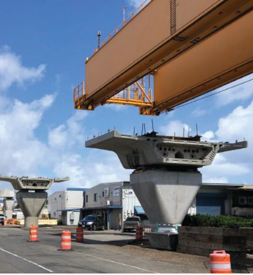
Figure 5. To accommodate overhead clearance requirements at Ualena Street, shallower-depth precast concrete guideway segments are used. Photo: Parsons Corporation.
