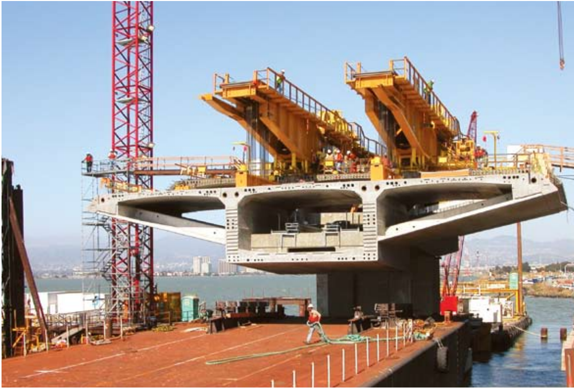
Two Self-Launching Erection Devices (above the deck), which are computerized beam-and-winch systems, lift segments from barges into place on the cantilevers.
