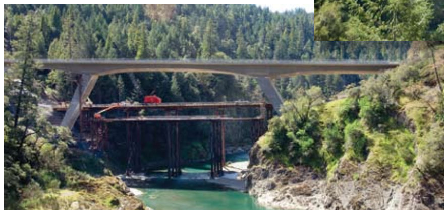
The north bridge, which is approximately 150 ft above the river, was built as a cast-on-falsework post-tensioned concrete box girder. The lower portion of the falsework (table top) can still be seen below the bridge as well as the temporary access trestle behind the bridge.
