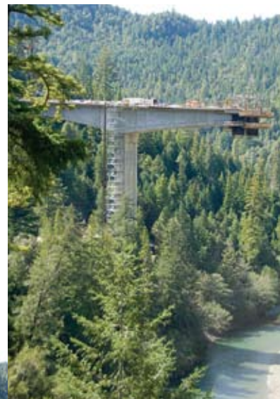
The south bridge, which is 275 ft above the river is a cast-in-place concrete segmental box girder constructed by the balanced cantilever method. Photos: © Jon Hirtz, Caltrans.
