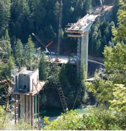
Looking south at segmental construction of the south bridge pier 2 cantilever with form travelers. Abutment 1 can be seen in the background. Photo: © Jon Hirtz, Caltrans.
