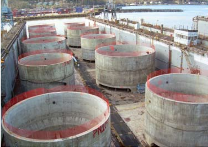
The 20 anchors built for the East half are 29 ft tall and range in diameter from 46 ft to 60 ft.
