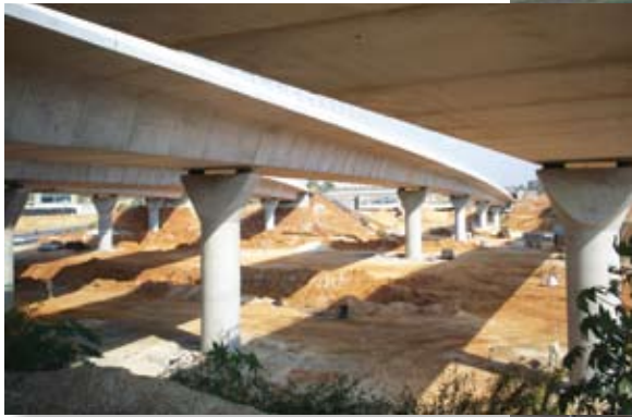
Longitudinal view of Bridge 22 on Road 431 in Israel, built in precast segmental cantilever construction. Photo: Finley Engineering Group Inc.
