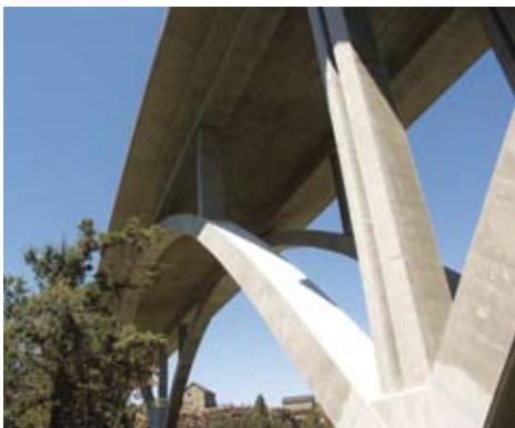
At the bents, each column pair appears as one column architecturally but operates as two columns functionally, with one of the pairs located on each side of the transverse deck joint. All photos: OBEC Consulting Engineers.
