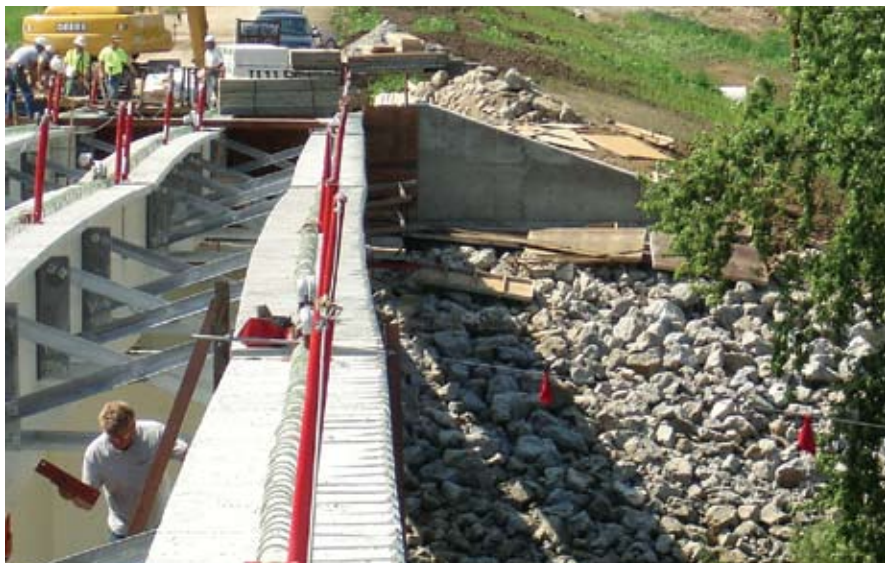
This photo shows long-term sweep. The LTS was subsequently removed by straightening, plumbing beam ends, and reattaching cross bracing to the straightened girders.
