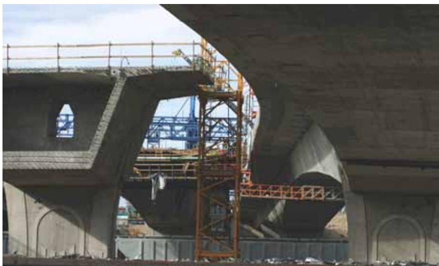
FINLEY is providing construction engineering for the 4th Street Bridge in Pueblo, Colo., which is being built over 28 active railroad tracks. Photo: Robert Heavilin, Flatiron Constructors Inc.
