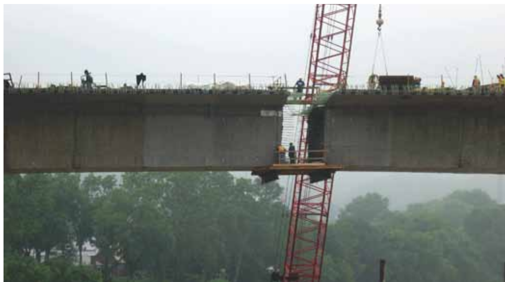
FINLEY served as construction engineering consultant on the I-64 Bridge over Kanawha River in Kanawha County, W.Va. The bridge features the longest concrete box-girder span in the United States at 760 ft, plus 460-ft and 540-ft side spans and five approach spans. Five piers are situated on land and two on the river's edge. Photo: Brayman Construction Corporation.
