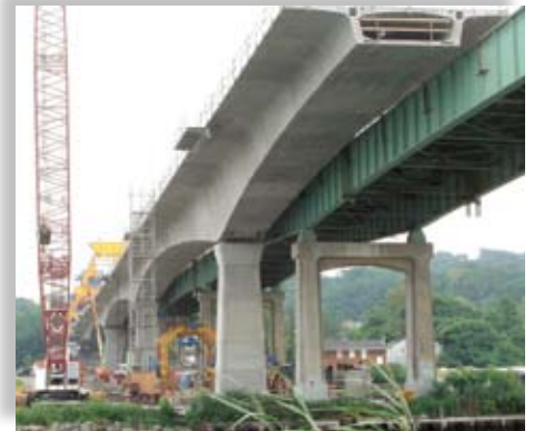
The Roslyn Viaduct Bridge on Route 25A over Hempstead Harbor, Long Island, N.Y. Photo: Rich Lorenzen.
