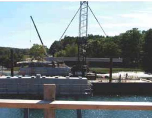
Beams were erected with a crane from jack-up barge on the York River.
