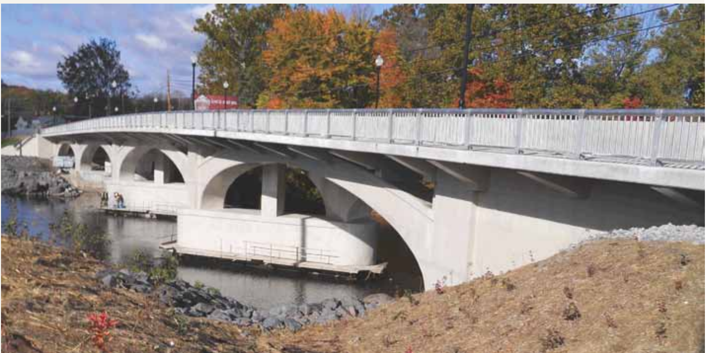
South elevation of the recently rehabilitated State Street Bridge over the Schuylkill River in Berks County, Pa. All photos: TranSystems.
