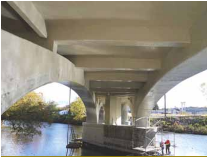
View of the underside of the rehabilitated bridge showing the original arches and the new cast-in-place concrete floor beams and deck.
