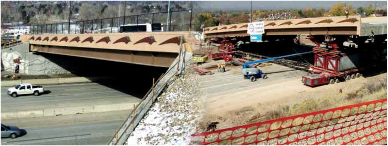
The 4500 South Bridge on State Route 266 in Salt Lake City, Utah, was removed and replaced in just 53 hours using self-propelled modular transporters. Photos: Utah Department of Transportation.
