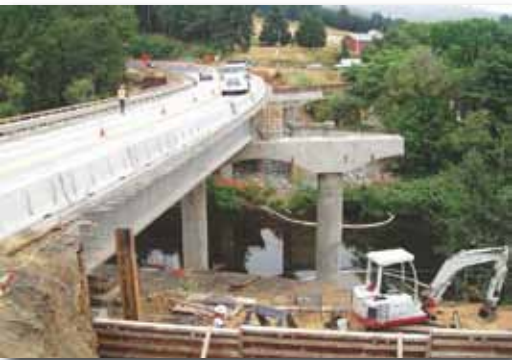
One of five crossings on an 11-mile-long stretch of OR 38 included in the Highways for LIFE Pilot Program. Precast concrete columns and piers were used to construct one-half of the bridge at a time. Photo: Oregon Department of Transportation.
