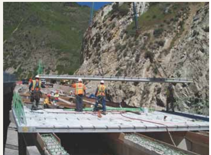
The panels were connected to the beams through reinforcing bars grouted into the top flanges of the beams. Photo: Utelite Corporation.
