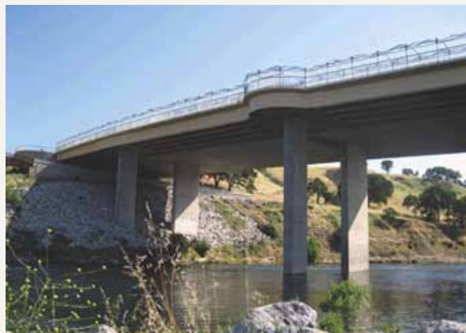
Hazel Avenue Bridge, a context sensitive solution, meeting public expectation and site constraints.
