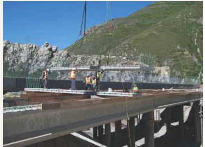
Lightweight concrete panels allowed the use of a thicker deck and overlay while not exceeding the capacity of the older beams. Photo: Utelite Corporation.
