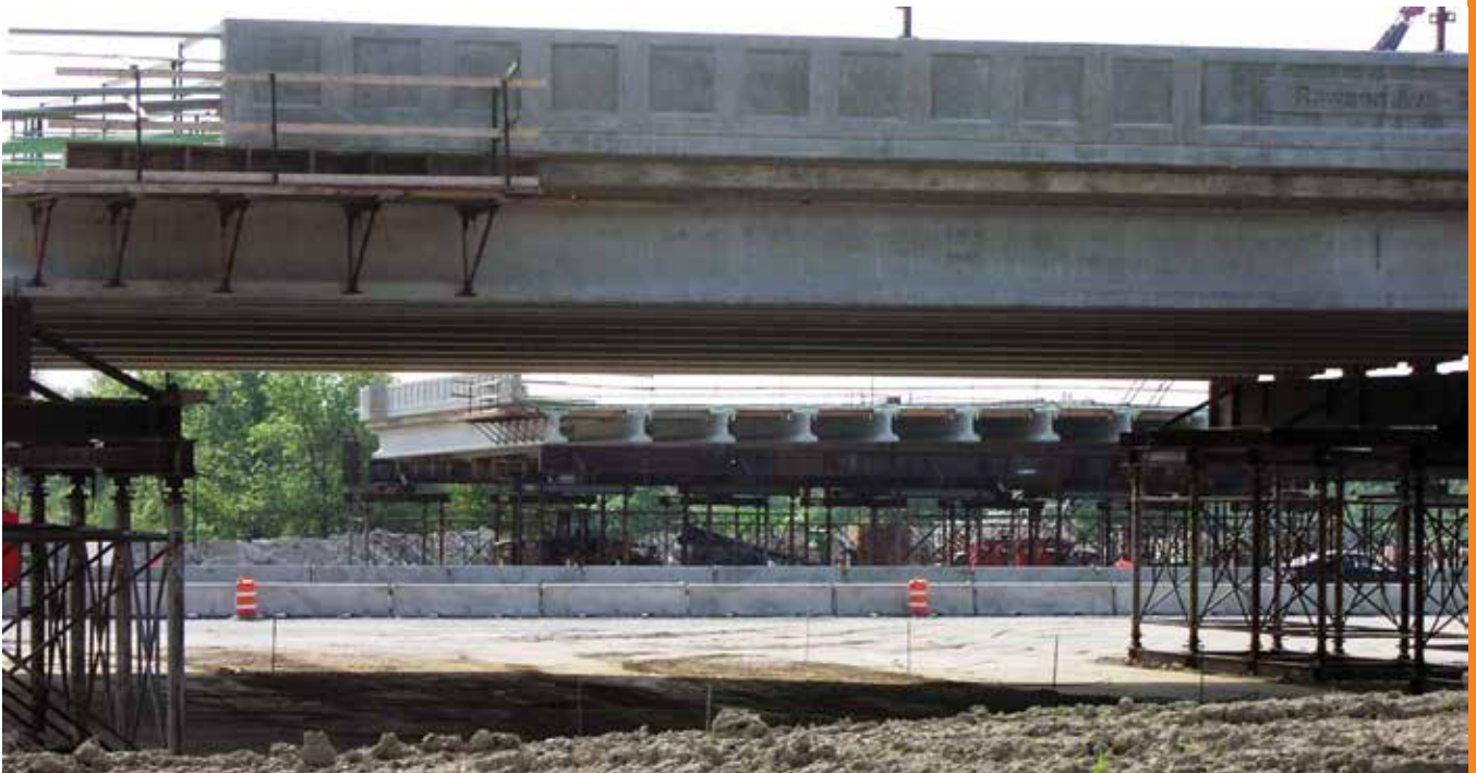
For the Rawson Avenue Bridge projects, the two spans were constructed on opposite sides of the expressway. Photo: Henry G. Russell Inc.
