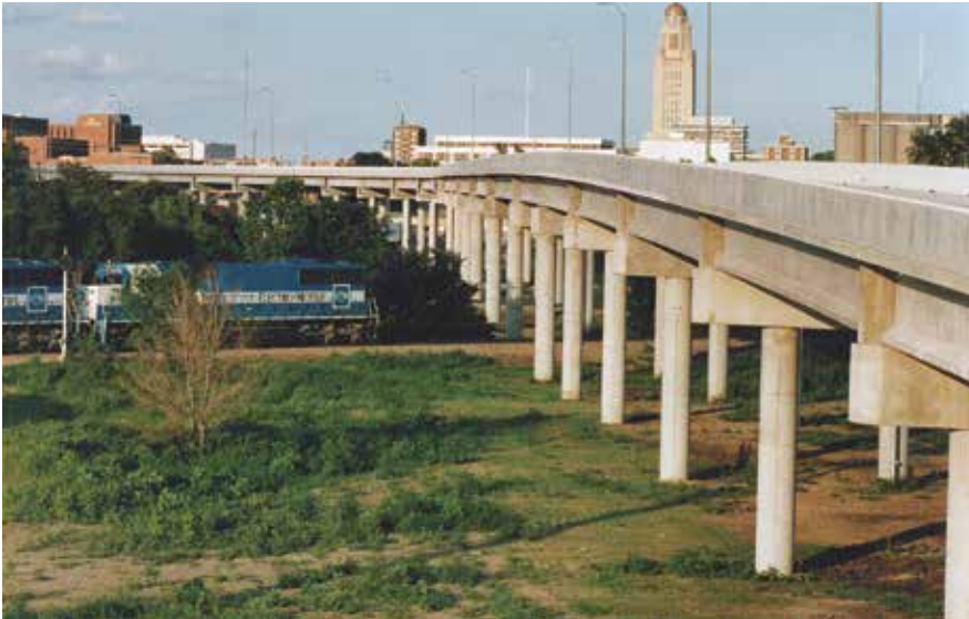
A 3200-ft-long, curved precast concrete solution eliminated multiple at-grade rail crossings at the Capitol Parkway West in Lincoln, Neb.
