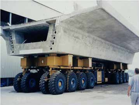
Full-span construction technique showing delivery of a prefabricated, simply supported box girder. Photo: SYSTRA.
