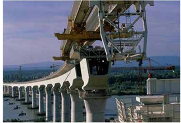
Avignon Viaducts during construction using precast concrete segments and a launching gantry.
