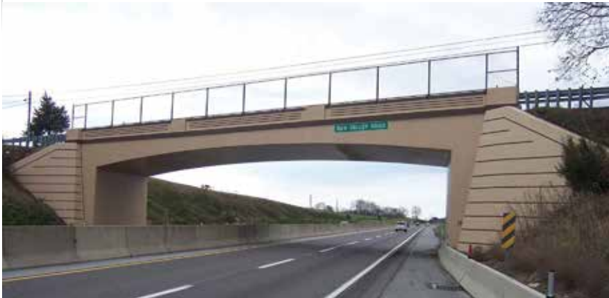
Typical reinforced concrete rigid frame bridge built in the 1930s. Preservation of this bridge was completed in 2010. All photos: Pennsylvania Turnpike Commission.
