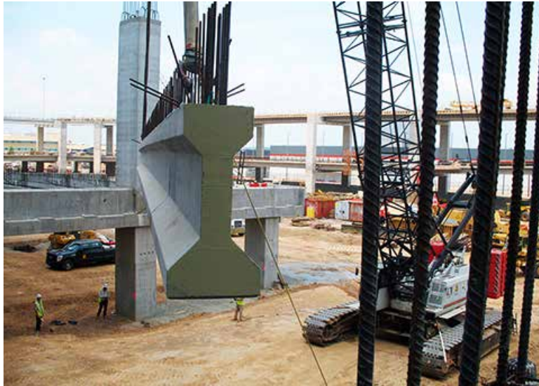
Nearly 600 AASHTO Type III concrete I-beams were used to construct the elevated roadway system. Photo: Max Anton Birnkammer.
