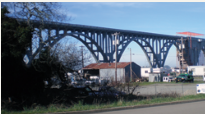
The Conde B. McCullough Bridge on Highway 101 at Coos Bay, Ore. Photo: International Concrete Repair Institute and BASF Corp.
