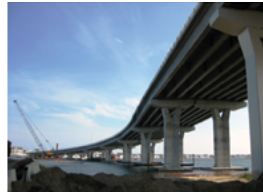
Underside of the Route 52 Bridge over the beach thoroughfare next to Ocean City.
