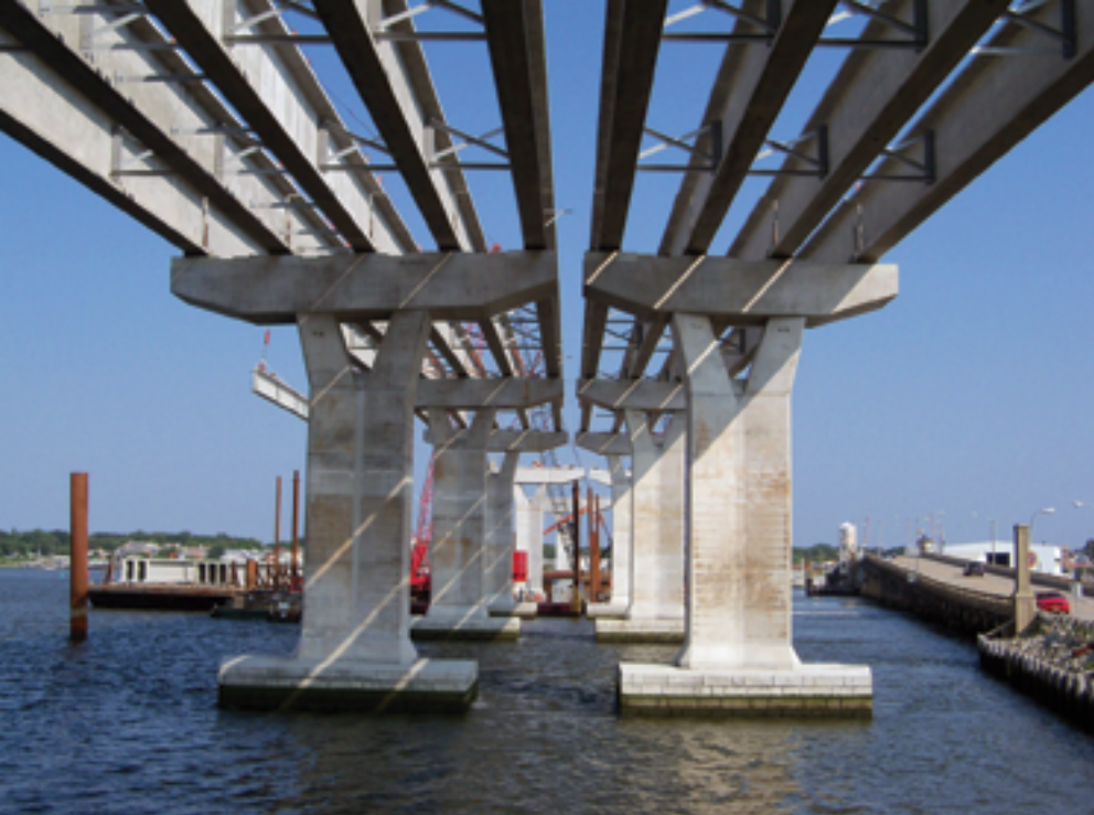
Route 52 Contract B: The prestressed bulb-tee beams are supported by the high level piers.
