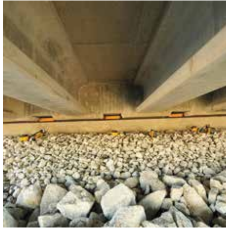
Preparing to lift the bridge superstructure with pancake jacks to remove the rollers. All Photos: Iowa Department of Transportation.
