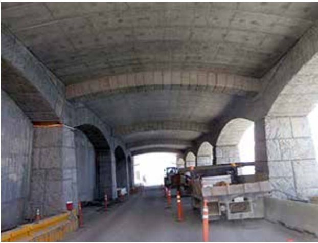
Interior view of the rock shed with roof panels in place, looking South.
