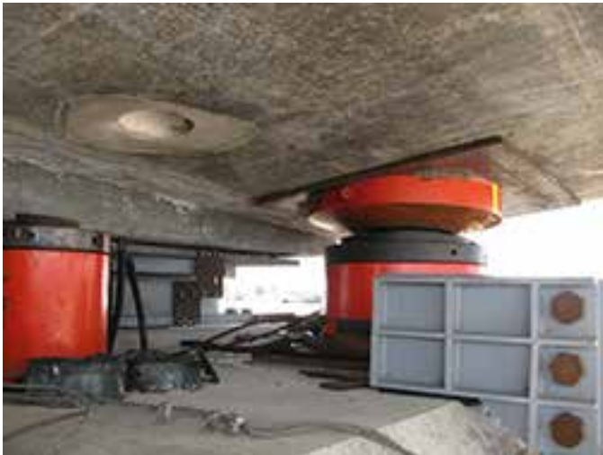
er cap / temporary erection jacks used on the Palmetto Interchange. Photo: Finley Engineering Group, Inc.
