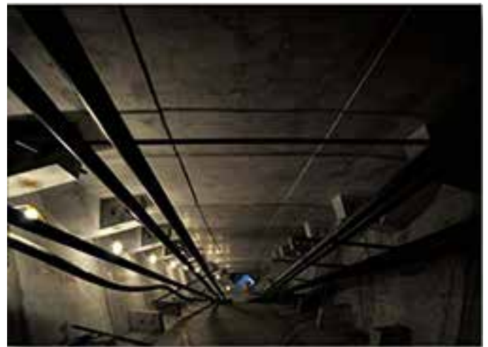
The use of external tendons also reduced maintenance costs by allowing improved access for future tendon replacement, upgrades and stressing of any single strand inside the box. Photo: Finley Engineering Group, Inc.
