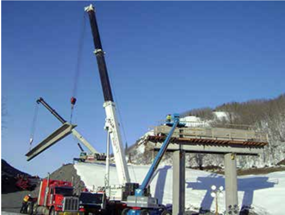
Picking a bulb-tee girder for winter construction of the Hicks Creek Bridge. All photos: Alaska Department of Transportation & Public Facilities.
