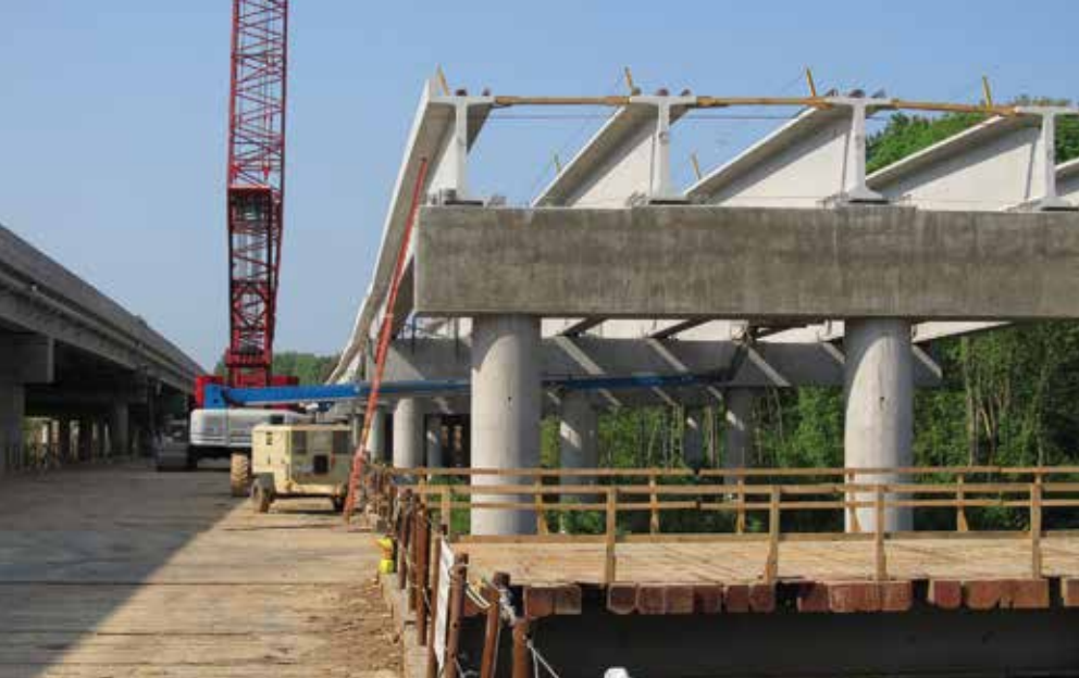
Erection of the southbound bridge, which is closely located next to the northbound bridge with the trestle between them. Photo: STV.
