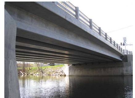
Figure 1. Ultra-high-performance concrete connections were used in the bridge over the Canandaigua Outlet in New York. Photo: Federal Highway Administration.
