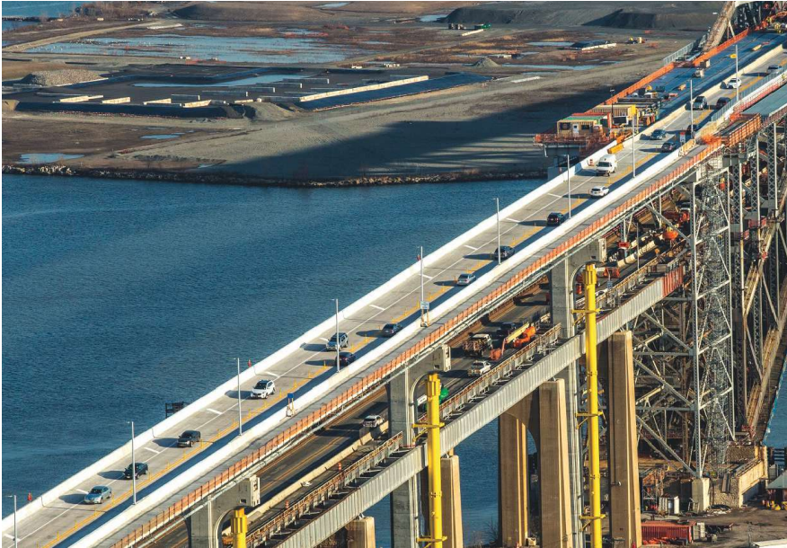
Traffic relocated to the new upper level of the Bayonne Bridge using the northbound approach structure. All Photos and Figures: HDR.
